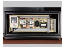
•INDEPENDENT DISTRIBUTION CABINET
